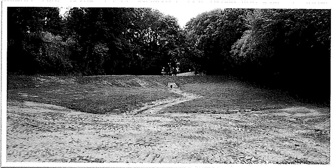
Looking south towards the substantially completed Area 1 lower bund. Grass seeding, flow control and grill to be fitted.
