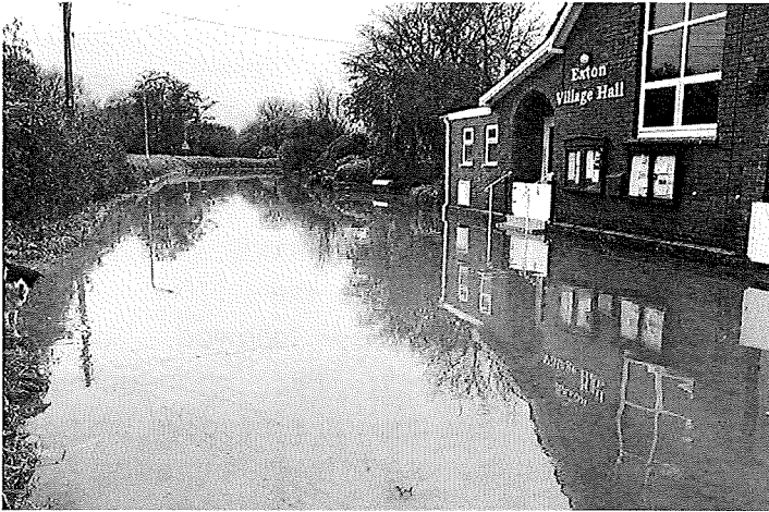
Flood Door Gates on Exton Village Hall, working to protect the hall in a surface water flood event. Source: Devon Live
