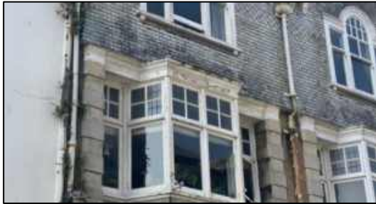
Maintenance required on the High Street.
